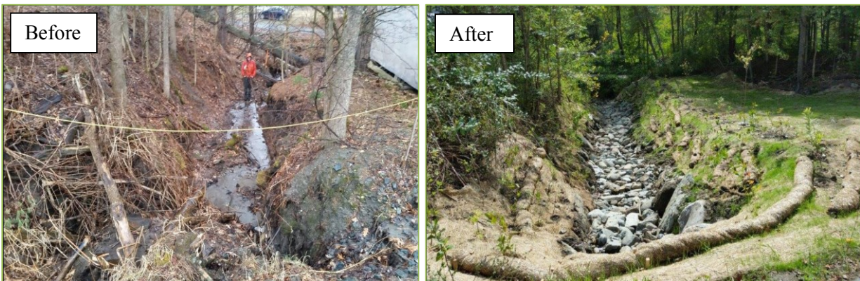
Gully restoration phase of a five part stormwater project to improve water quality in Centerville Brook in Hyde Park.
