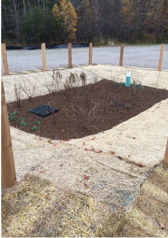
Figure 1. Lake Iroquois Recreation District bioretention basin
