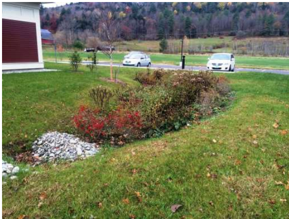
One of five rain garden pockets installed at the Waitsfield town offices to treat impervious surfaces.
