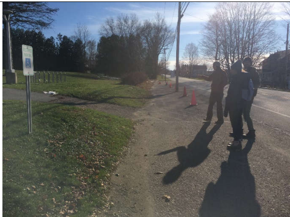
Photo 1: Accumulated sediment suggests water pools and evaporates in the handicap parking area.
