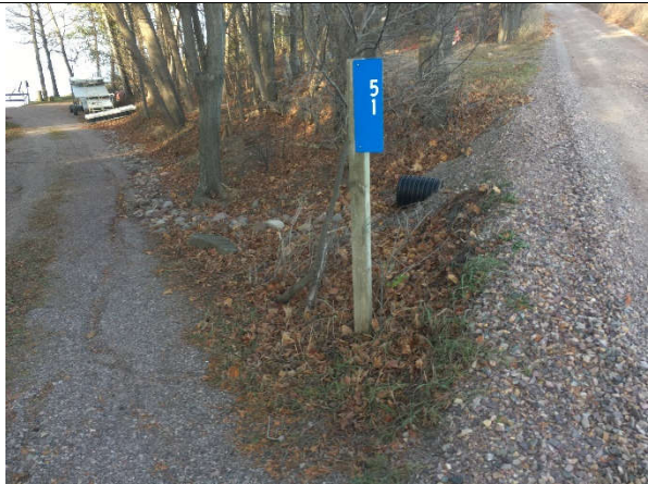
Photo 1: Erosion down driveway (left). Cross culvert outlet with stone stabilization (right).
