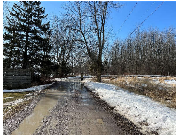
Photo 2: Ponded water on Lombard Lane. The Cross-culvert is located at the bend in the road.
