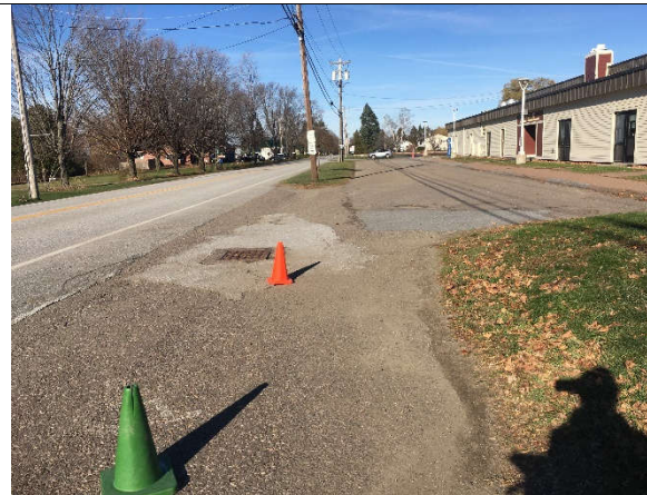
Photo 2: The catch basin is completely full of sediment and higher than the handicap parking area.
