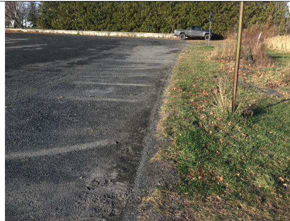
Photo 2: Grass between parking lot and wetland with accumulated sediment.
