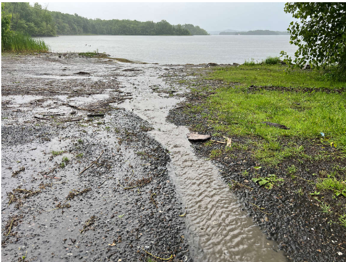
Figure 6: Runoff from the gravel parking area at the VT Fish & Wildlife Boat Launch. The concept design for this area describes BMPs that would slow and treat stormwater runoff and reestablish native vegetation along the lakeshore.
