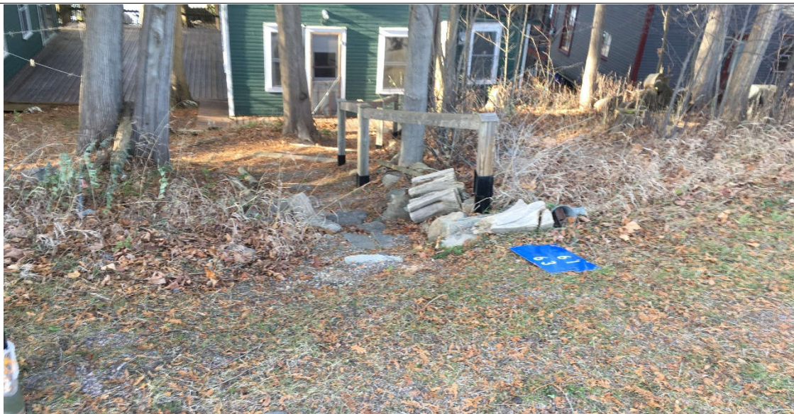
Photo 1: Runoff from road and lawn conveys sediment down existing steps.
