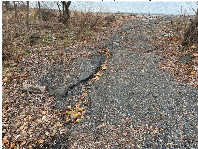
Photo 1: Gully erosion on ramp down to the lake
