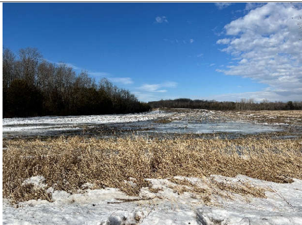
Photo 1: Agricultural runoff concentrates to a cross-culvert on Lombard Lane.
