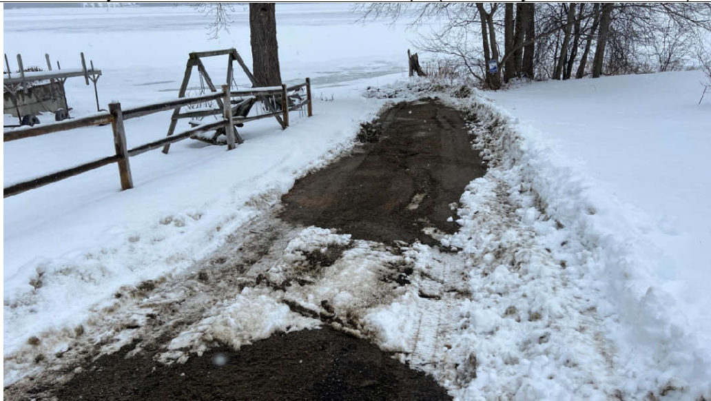
Photo 1: Ramp on Lavigne Road with erosion down to lake
