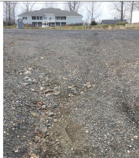
Photo 2: Erosion on the boat ramp
