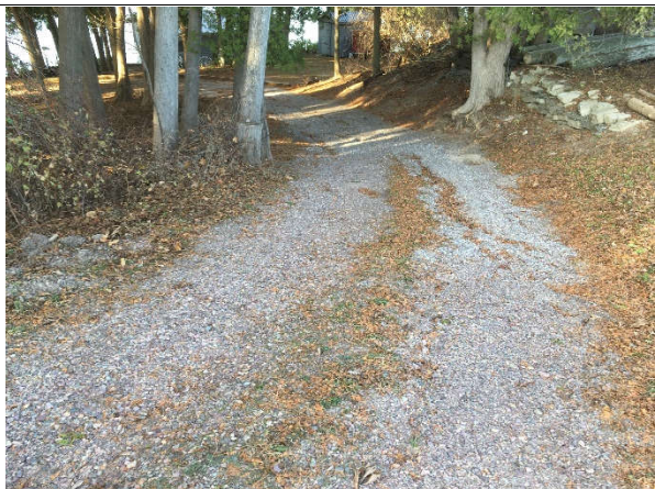
Photo 1: Rill erosion caused by runoff down driveway.
